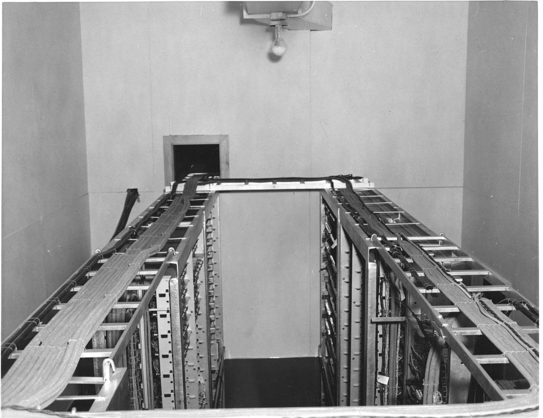
CABLE RACKS WITH CABLES, KELLOGG 7-2 X-BAR, EDWARDS AIR FORCE BASE, DOUGLAS AIRCRAFT, CA 1955
