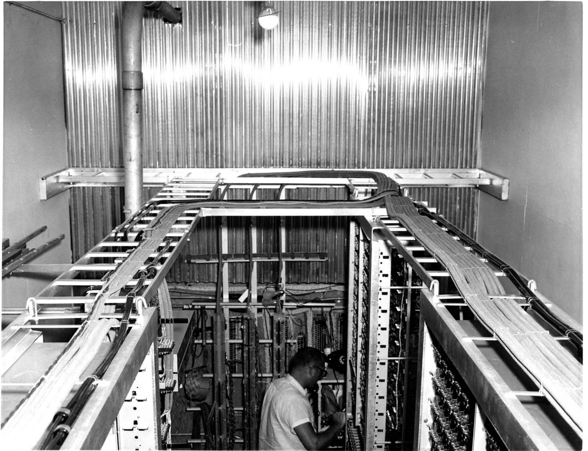
CABLE RACK WITH SEWED CABLES, ODIS LEVRIER TESTING KELLOGG 7-2, X-BAR, EDWARDS AIR FORCE BASE, DOUGLAS AIRCRAFT, CA 1955
