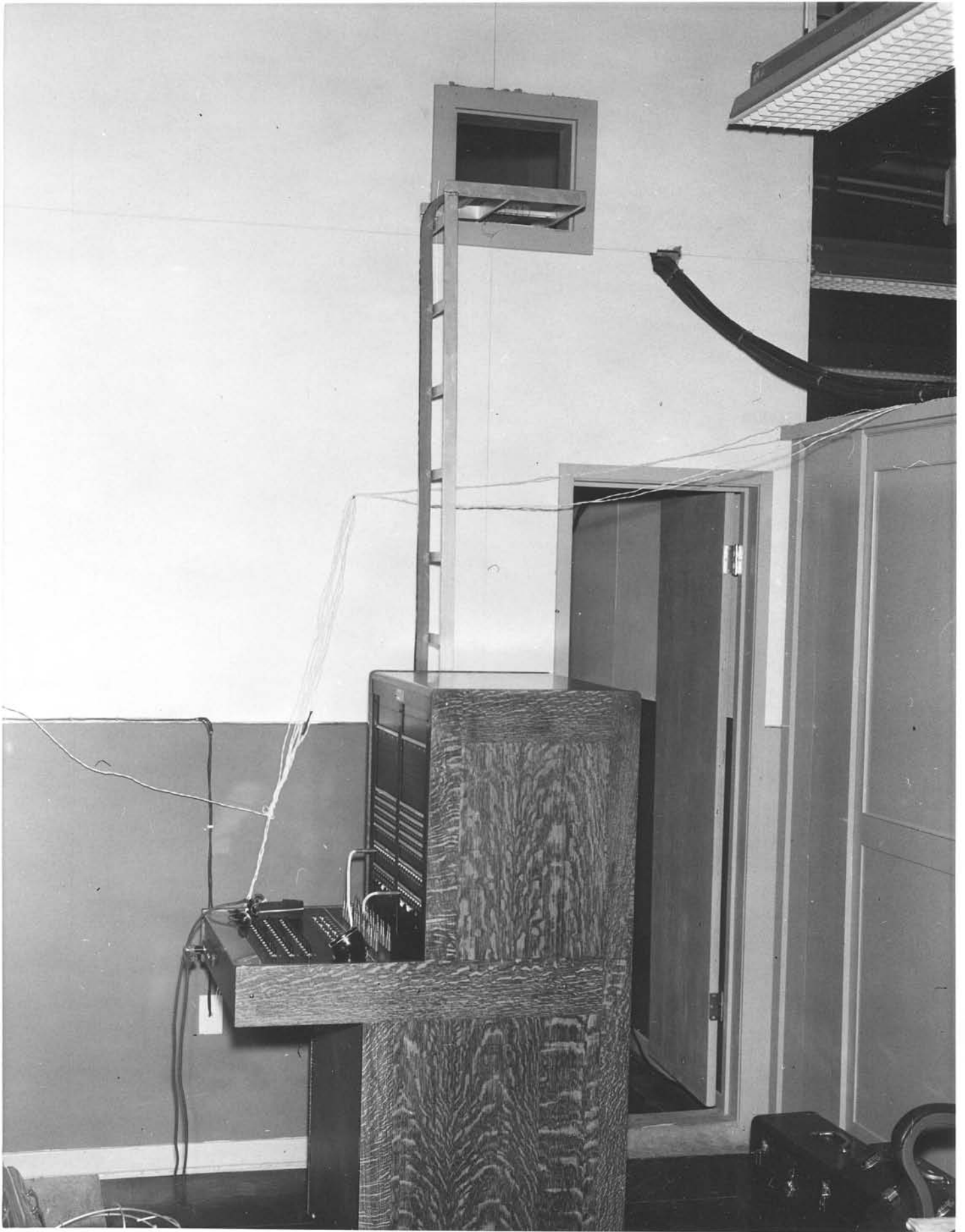
KELLOGG ATTENDANTS SWITCHBOARD, KELLOGG 7-2 X-BAR, EDWARDS AIR FORCE BASE, DOUGLAS AIRCRAFT, CA 1955
