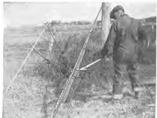
For taking up slack in guy wire a No. 325 is speedy and efficient
