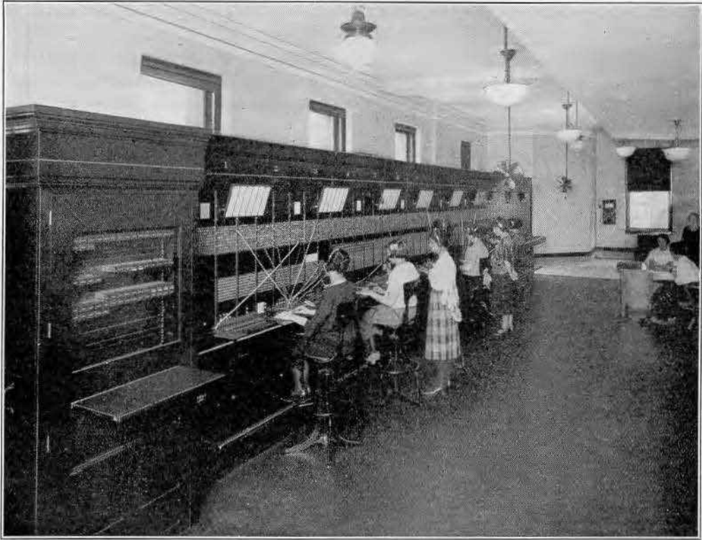
Operating Room Showing Main Switchboard and Chief Operator's Desk
