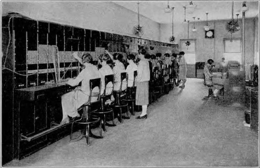
No. 11 Multiple Switchboard in Operation
